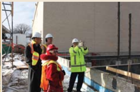
HLC Project Manager Bill Myers (right) explains construction progress to MP Brandon East Drew Caldwell (left) and Manitoba Premier Greg Selinger (back centre) as Dr Poff (front centre) looks on.
